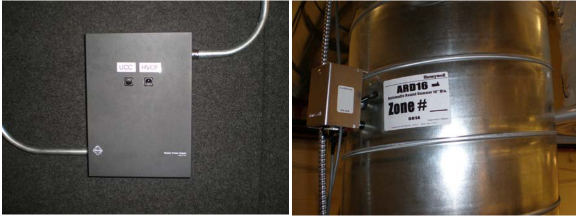
Figure 22. Electric damper switch and actuator.
